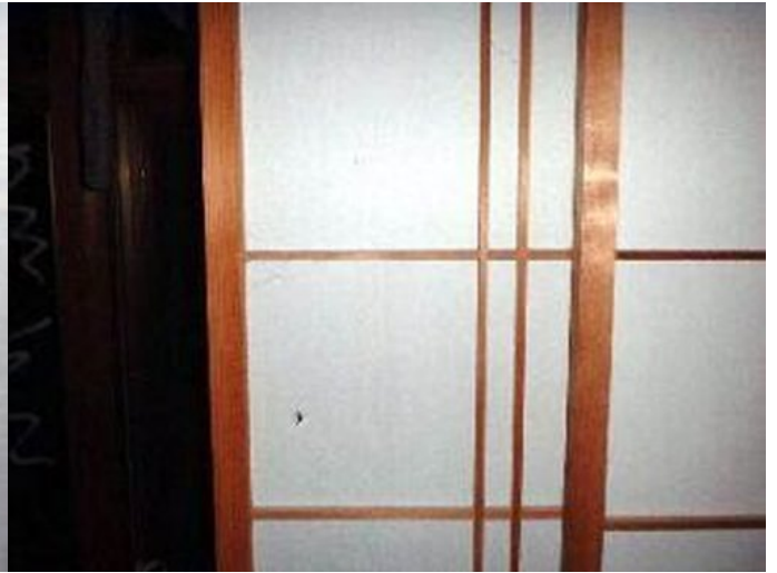
Typical hole in shoji door
